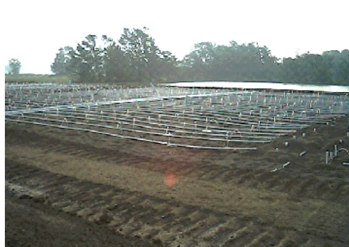
new system flooding.....
